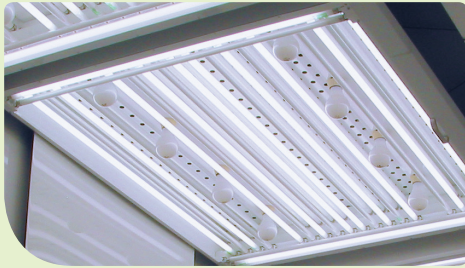
T5 FLUORESCENT LIGHTING
